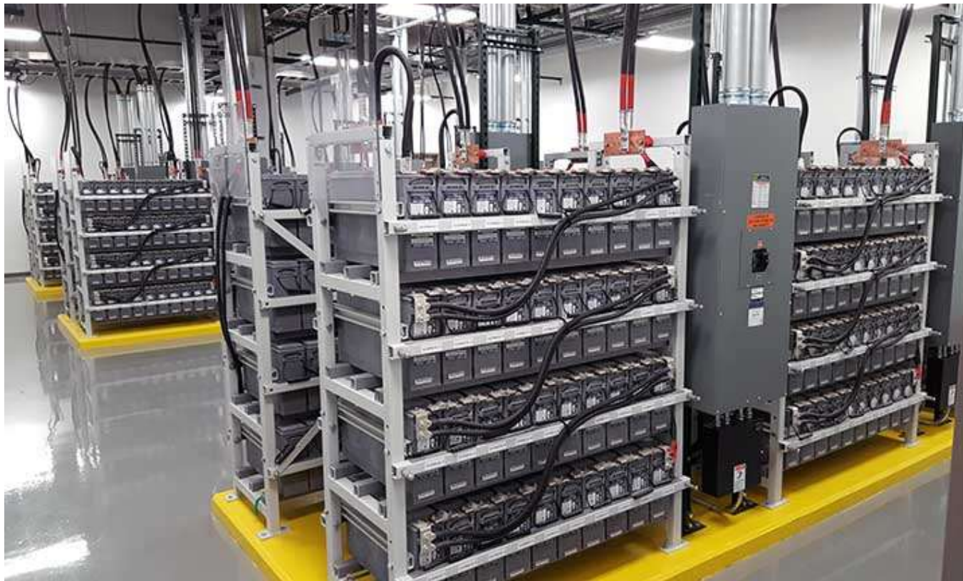
A battery room inside a data center campus in Richmond, VA. These batteries provide temporary emergency power for UPS systems. (Photo: Rich Miller)
